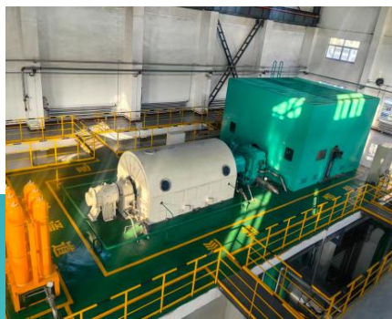
Caption: Huasheng Chemical's new waste heat power generation unit
